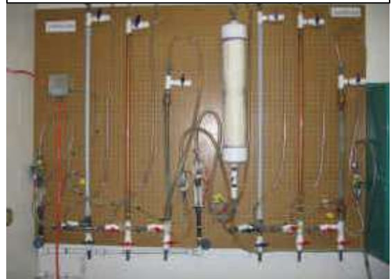
FIGURE 5 Pipe Loop Apparatus for Corrosion Control Pilot Test
