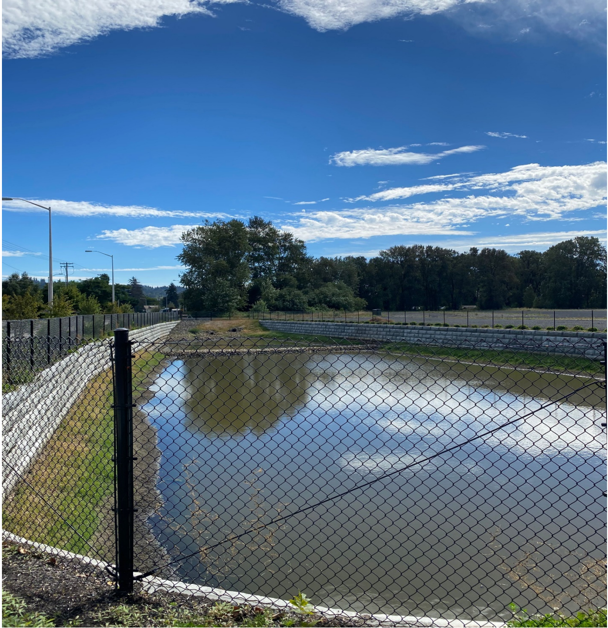
Storm water facility constructed along Goerig Slough through neighboring development(s) to the East of development
