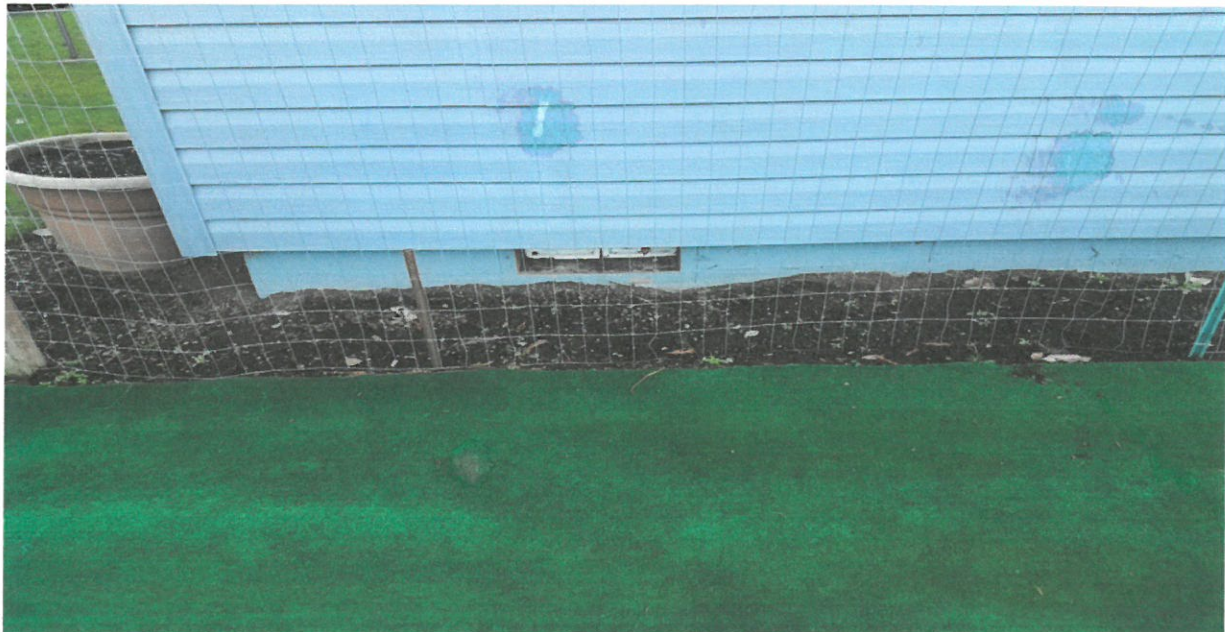
Photo Two Caption: Picture shows typical vent on back of house at Northeast corner. Photo taken 12/20/2017.
