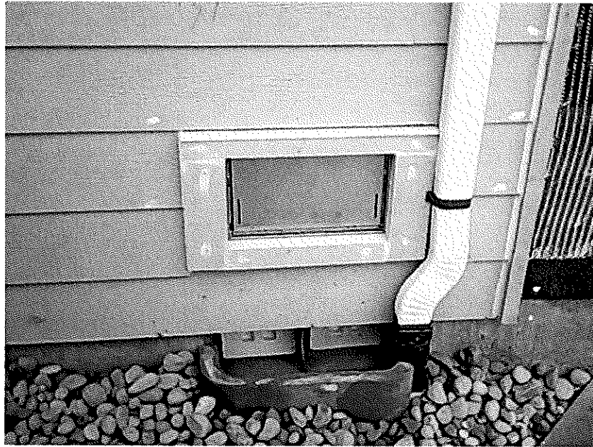
FLOOD OPENING IN GARAGE 12/09/2013
