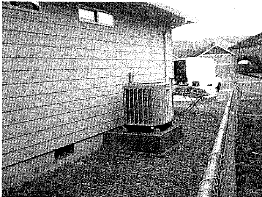
SIDE OF HOUSE WITH HEAT PUMP 12/05/2013
