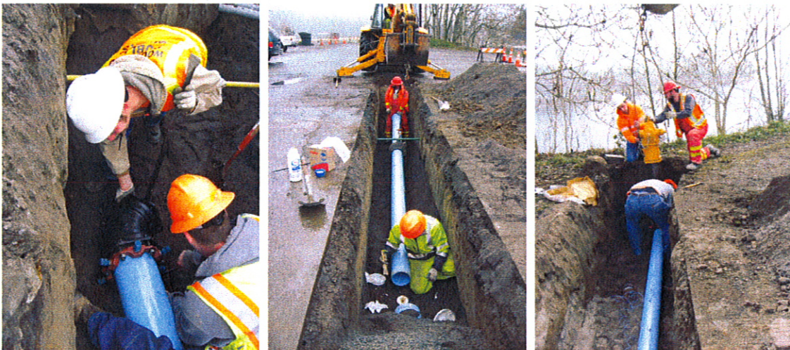
Davidson Alley Water Line Installation From 2nd Street to Goerig Street behind Swanson Plaza
