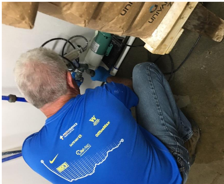
BRUCE SLONIKER REPLACED MAG PUMP ON SODA ASH MACHINE WTP
